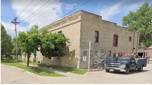
Building A. This building was the base of field operations for the water field crews. It currently serves as the Water stores building
